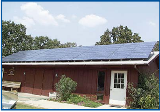
Solar system installed at the Heifer Ranch in Perryville, Arkansas. Photo courtesy of NREL.
