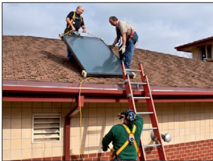
Installing a flat plate solar water heating collector. Photo: Courtesy of National Renewable Energy Laboratory
