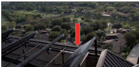
Solar collectors installed too close together, causing winter shading. Photo: Thomas Isaac, courtesy of Techsun Solar, Inc.
