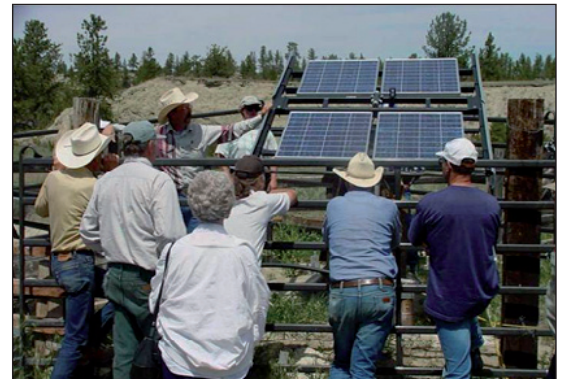
This 320-watt PV system in Montana pumps 5.5 gallons per minute from a 65-foot deep well, delivering enough water to meet the needs of 100 cow-calf pairs. The cost of its solar components was $5,500. Photo: Mike Morris, NCAT
