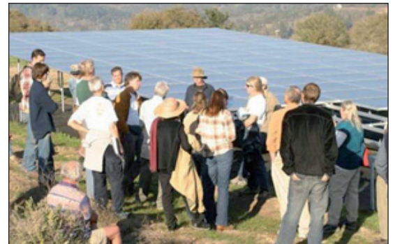
This large 15-kilowatt solar array meets 80% of the electrical demand at an organic vegetable farm in California and was installed at a cost of $90,000 (after all incentives), despite having a long payback period of more than 20 years. Photo: Mike Morris, NCAT
