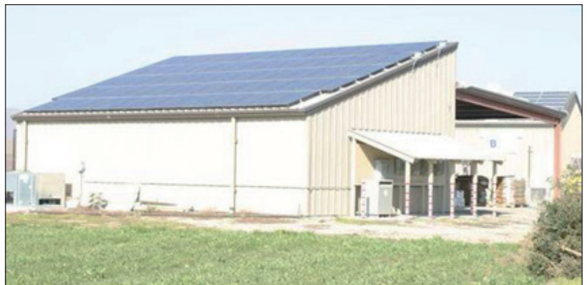
Solar arrays generating 10.8 kilowatts and 12.6 kilowatts greet visitors to this California organic vegetable farm. The arrays meet 25% of the farm's electrical energy needs. Photo: Mike Morris, NCAAT
