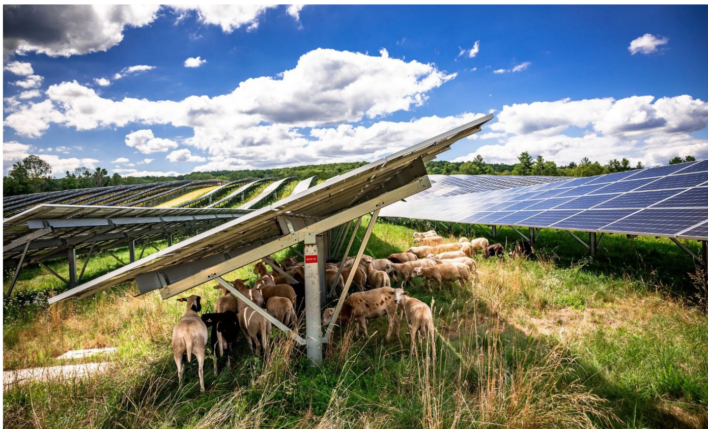
Sheep grazing in the shade of solar panels. Photo: NCAT
