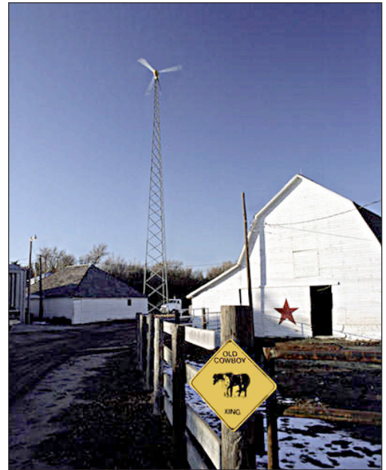
Small wind turbines can provide supplemental power for farms and ranches, as on this farm in western Kansas. Excess power is fed back into the utility grid. Photo: Warren Gretz, NREL/PIX09615
