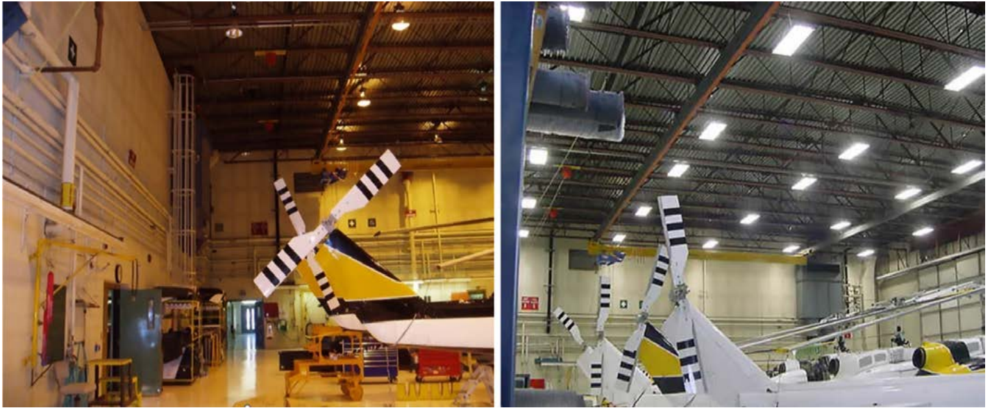
Figure 9. Lighting retrofit to LEDs with improved color rendering, efficacy, and efficiency. Photos: NCAT
