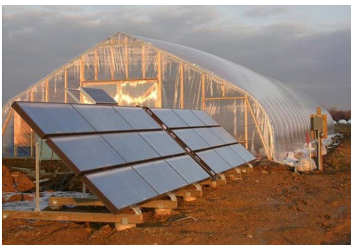
Solar thermal flat-plate collectors heating a high tunnel. Photo: NCAT
