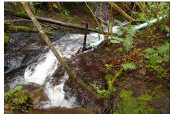
A micro-hydro intake and penstock temporarily divert a portion of the water flow and carry it to the location of the turbine. Photo: Leif Kindberg, NCAT
