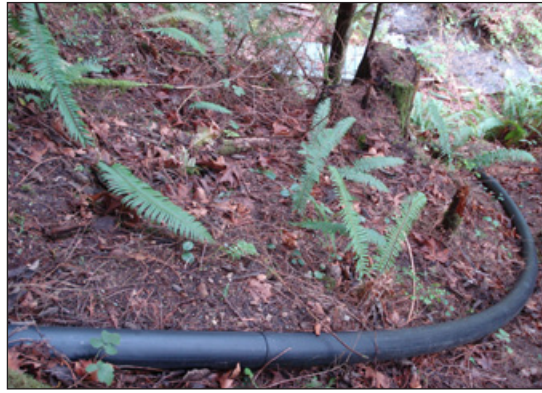
The penstock is sized and selected for each site. Often, a pressure-rated steel or plastic pipe is used. Photo: Leif Kindberg, NCAT
