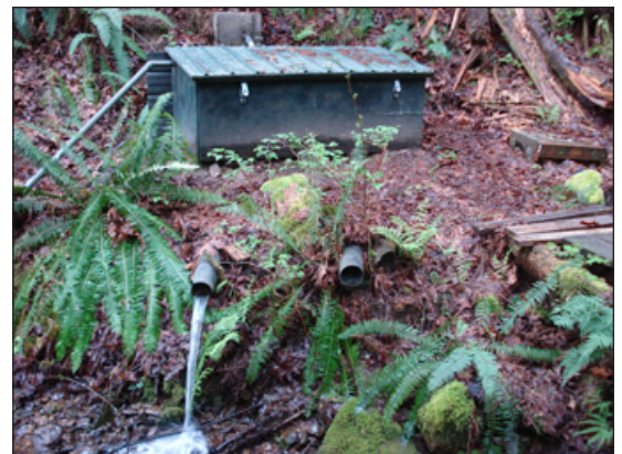
A “run-of-river” system returns flow to the same stream, reduces environmental impact, and generally eases the permitting process. Photo: Leif Kindberg, NCAT
