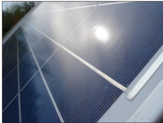
Energy alternatives like solar are not constant—unlike many micro-hydro projects that can operate 24/7—but may be a better choice depending on the project site and power needs. Photo: Leif Kindberg, NCAT
