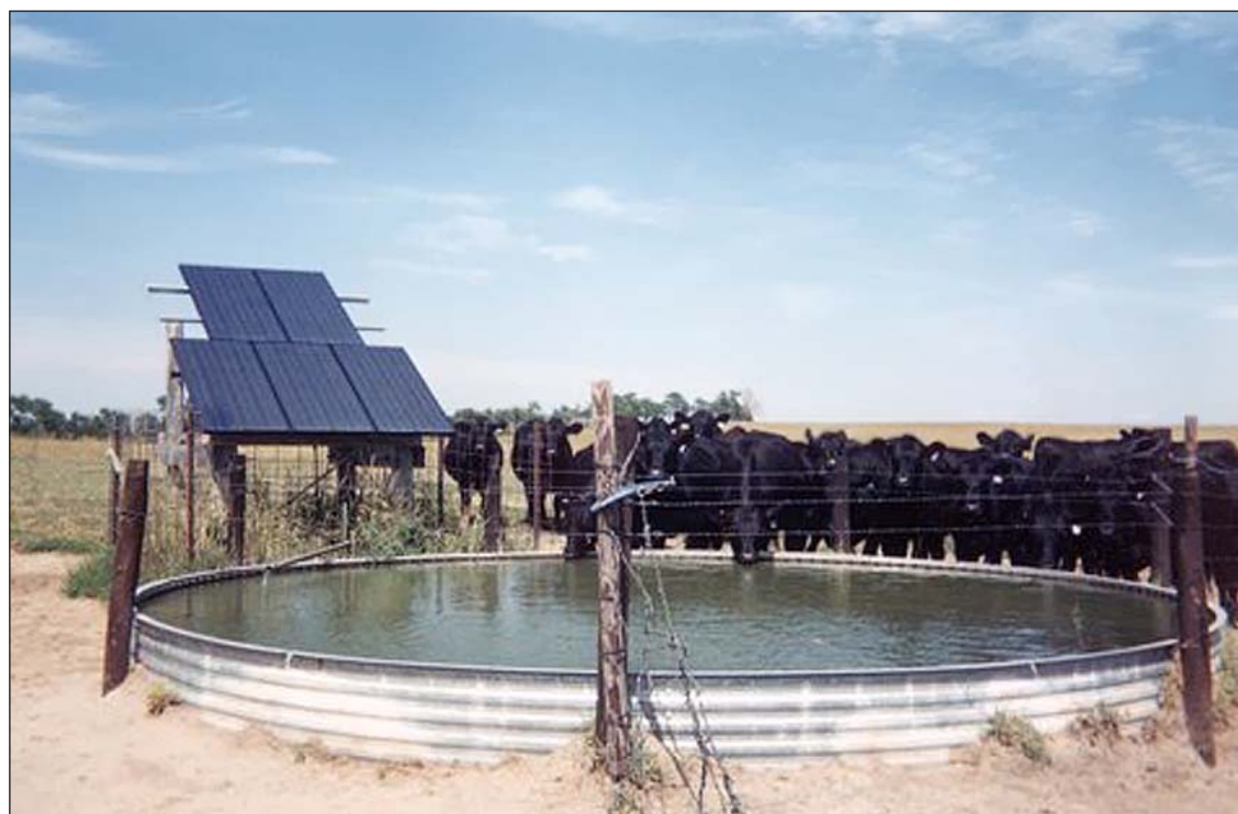
Solar-powered livestock watering system. Photo: NREL
